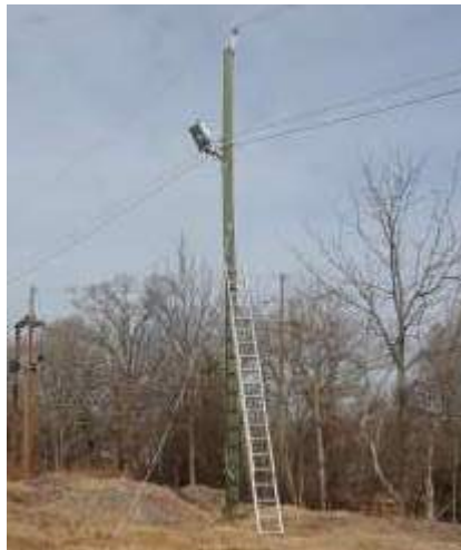
Antenna attached to a light pole.
